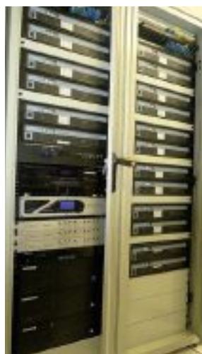
An audio EQ rack with MTS amplifiers, MediaMatrix Nion NX DSP and ION 8.8 COMS
